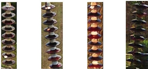
Figure 6. Damaged Insulator Examples Imagined by PGANs
